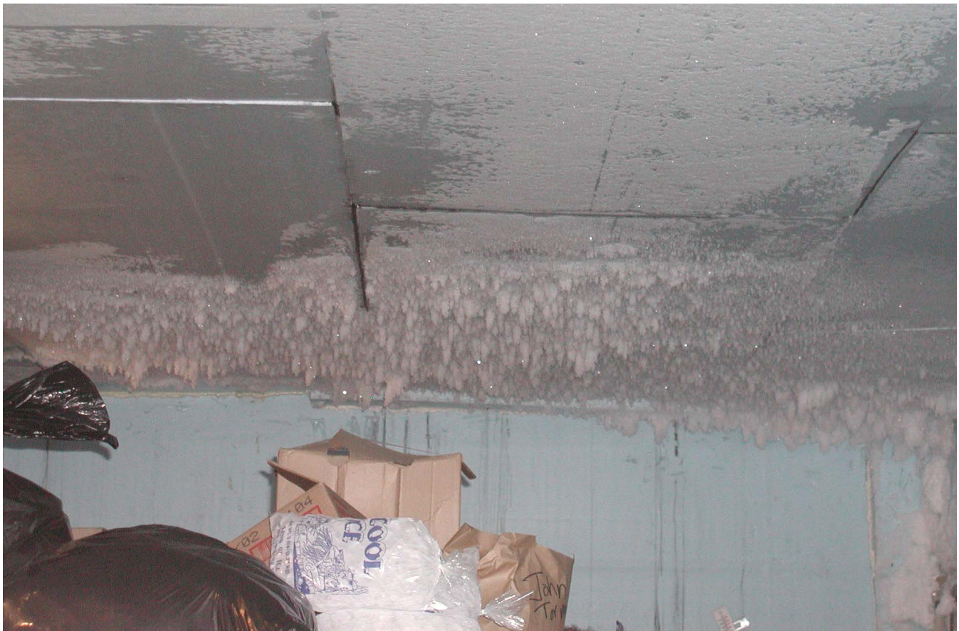
Condensate on the ceiling of a cooler can drip onto contents below, creating a food safety risk.
